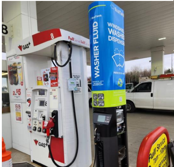
Figure A 1: An EcoTank windshield washer fluid dispenser installed at a Canadian Tire Gas+ gas bar.
