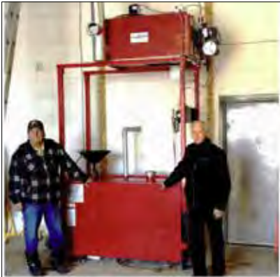
Ron Benson, Executive Director of MARRC with Solomon Mason, Project Manager with St. Theresa Point standing in front of the used oil burner installed at the Fire Station.
